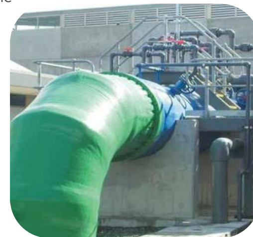
Seawater Desalination Plant
