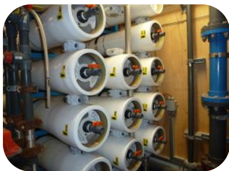
Reverse Osmosis racks
