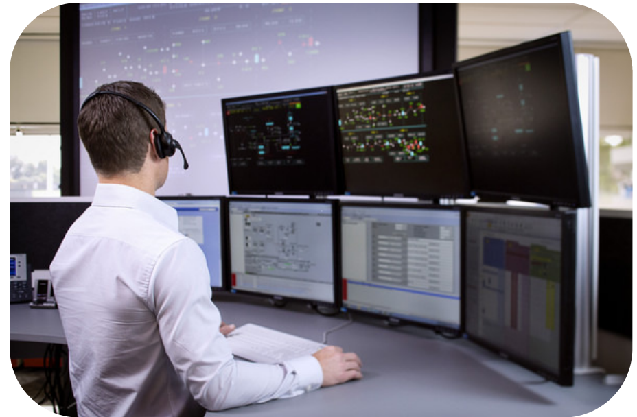
Operation centre monitoring alarms
