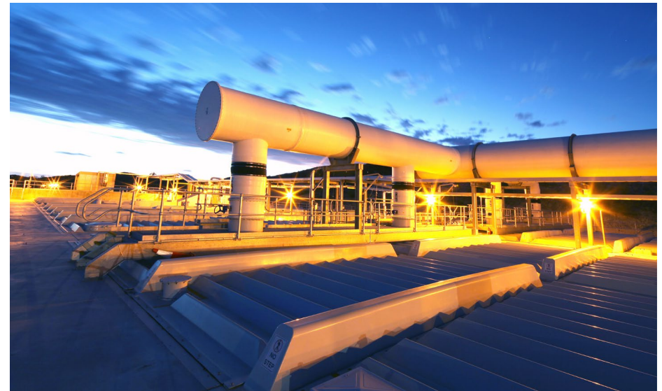
Figure 24: Alkimos WWTP odour control
