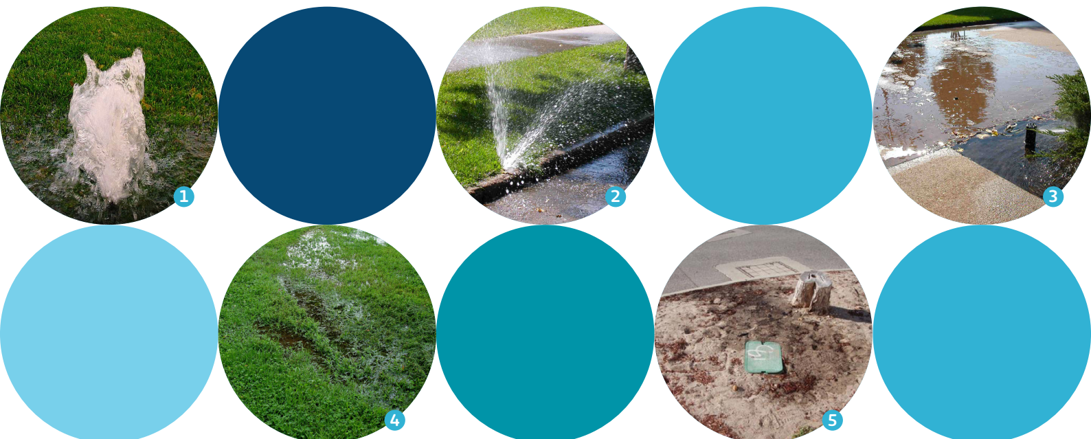
1. Broken sprinkler 2. Broken irrigation pipe 3. Broken irrigation pipe 4. Inundated water caused by broken irrigation pipes 5. Leaking solenoid
